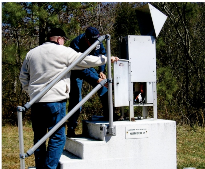
Figure 3.13. East Tennessee Technology Park ambient air monitoring station
